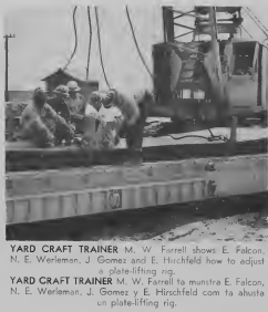
YARD CRAFT TRAINER M. W. Farrell shows E. Falcon, N. E. Werleman, J. Gomez and E. Hirschfeld how to adjust a plate-lifting rig. YARD CRAFT TRAINER M. W. Farrell ta munstra E. Falcon, N. E. Werleman, J. Gomez y E. Hirschfeld con ta abusta un plate-lifting rig.
